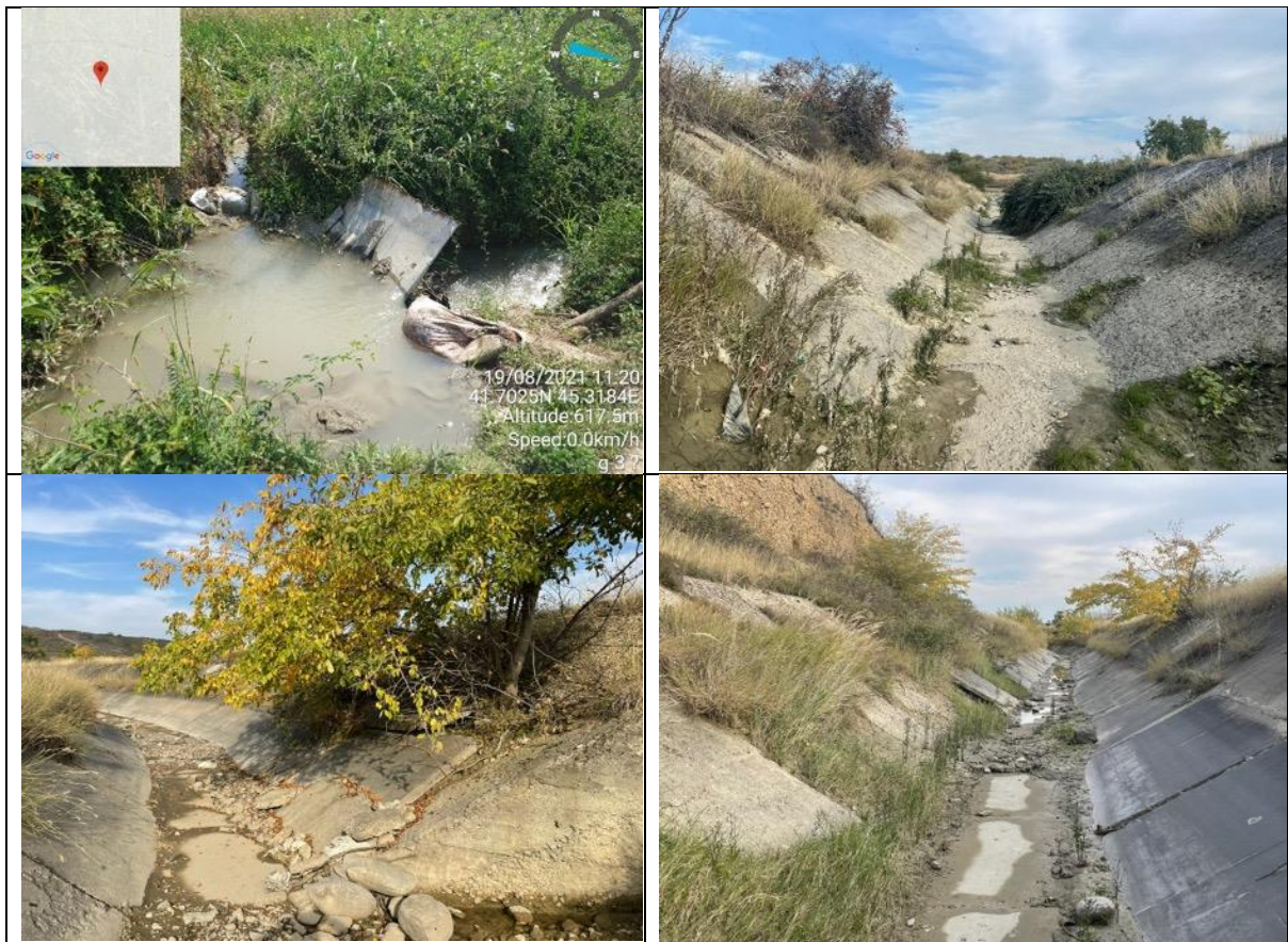
Source of photos: Report: Left Main Canal of Kverno Samgor Irrigation System (From Pk. 0+00 To Pk. 488+50= First Line (And Other) Distribution Branches (G-1-G42) Inventory . Ta-54014-002 GEO: Preparing the Water Resources Sector Development Program – Project Design Consultants.
