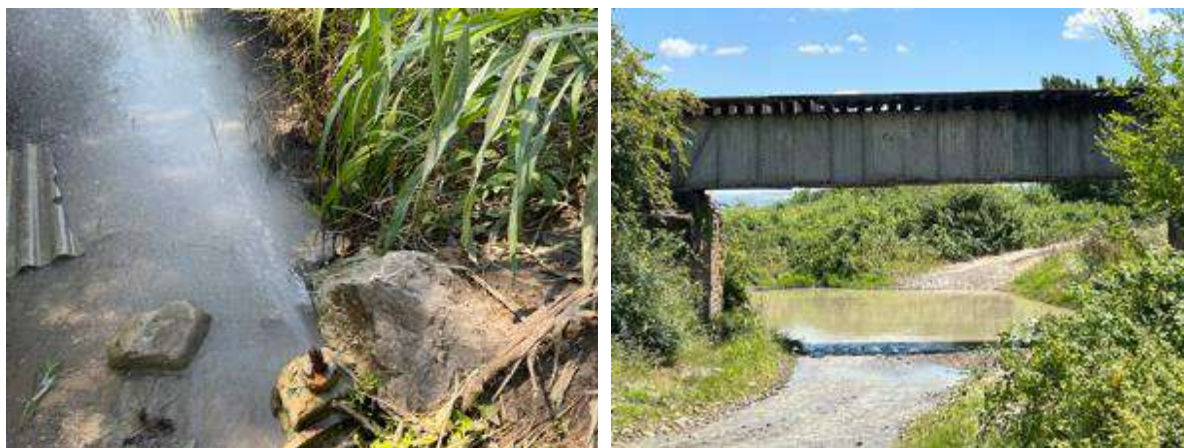
Figure 31: Leakages due to damaged system
